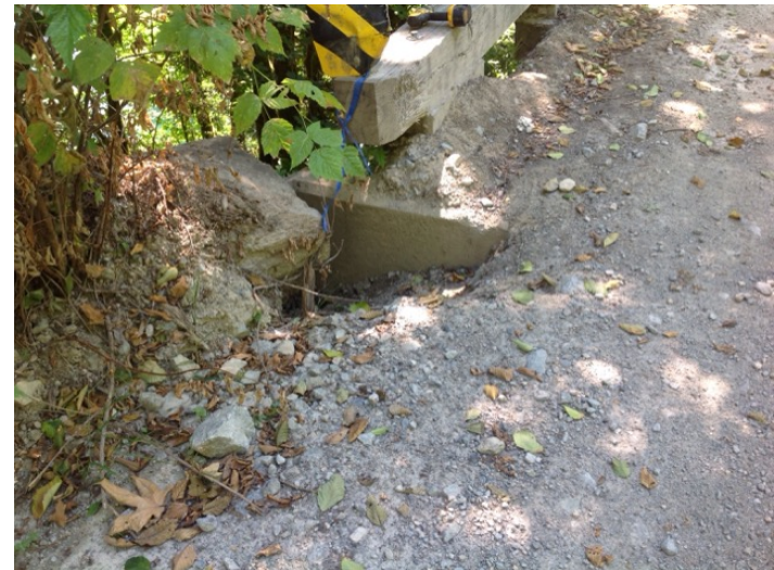
eroding fill left downstream approach
