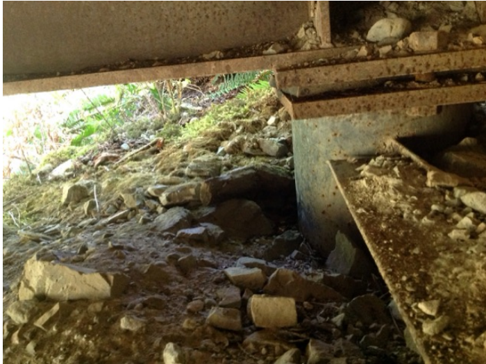
bulging pads - off centre plates
